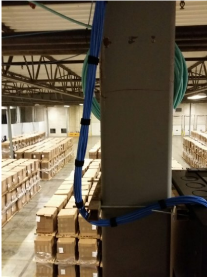
Side view of pole mounted cabinet using Unistrut and treaded rod
