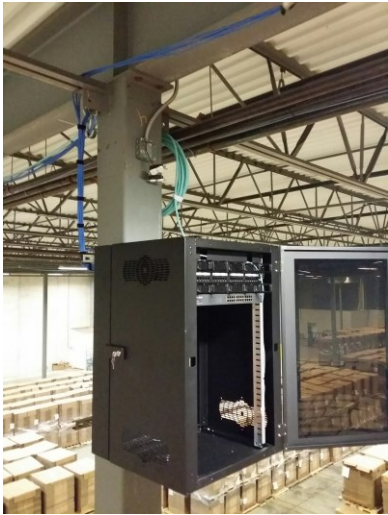
Front view of pole mounted cabinet
