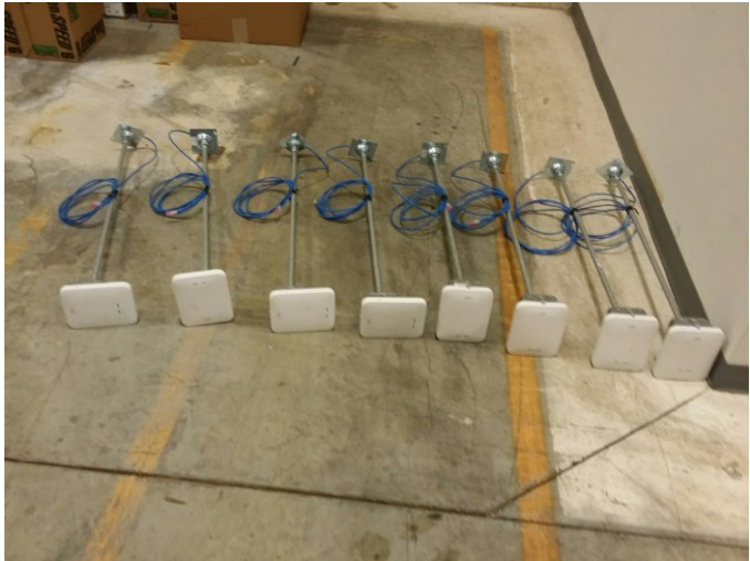
Drop Pole Assemblies with AP mounted
