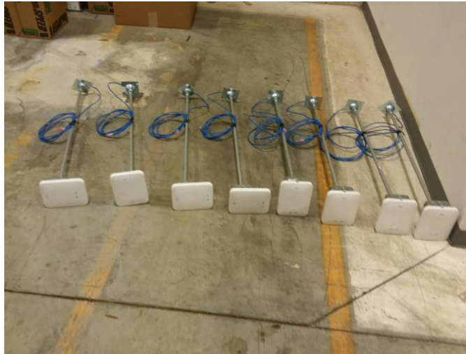
Drop Pole Assemblies with AP mounted
